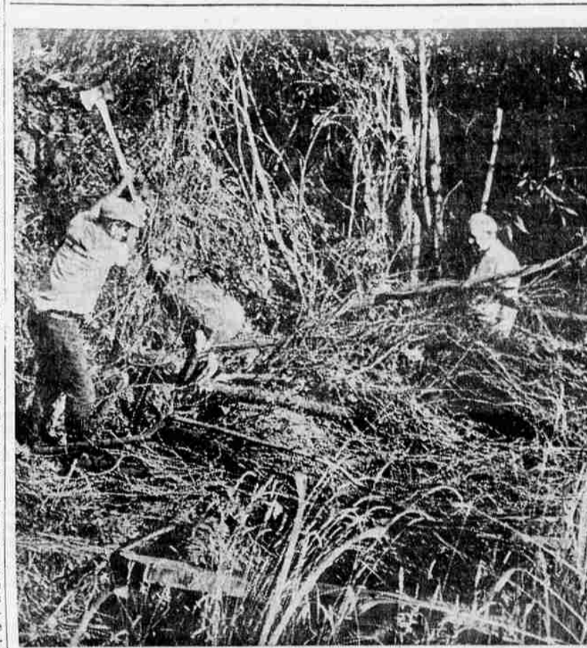
OPERATION CLEARANCE—Transients booked on vagrancy charges are put to task of leveling their woody homes in "hobo jungle" area, along railroad tracks just south of Franklin Ave. A 14-man crew has been busy this week clearing trees and brush growing along irrigation canal, abreast of Oregon Trail Box factory. Supervising police officer Maurice Ries says vagrants are hard workers and quite cooperative.
