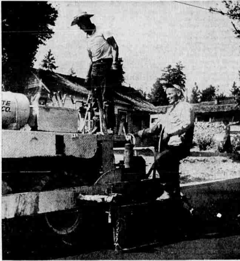
PAVED AT LAST — Two-inch layer of asphalt surfacing is laid over three-block strip of roadway at W. 11th Street, Newport to Quincy, by workmen of Bend Aggregate & Paving Company. Roadway was paved Thursday and ready for motoring travel this morning. Project is first actual paving operation in Bend in two years. Portions of three other Bend streets — E. Seward, E. Kearney, and E. Lafayette Avenues, are scheduled for paving within a week. Pictured above are driver Ted Lewis, left, and Oliver Fraser.
