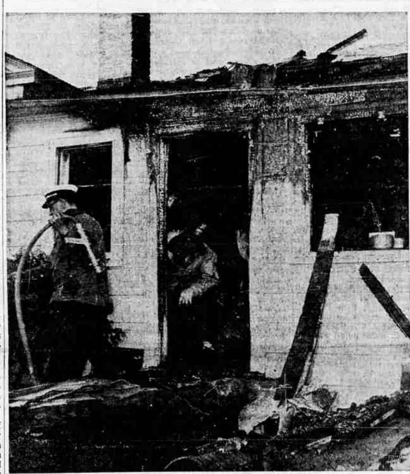
FIRE DAMAGES BEND HOME — The home of Mrs. Otto Larson, 64 Gilchrist, was extensively damaged by fire early this morning in which Mrs. Larson suffered a foot burn. Pictured here are firemen who were back on the job later this morning when embers started smoking. Left, carrying hose, Captain Orval E. Johnson, Bend fireman. Norman Wells is shown coming under barrier.
