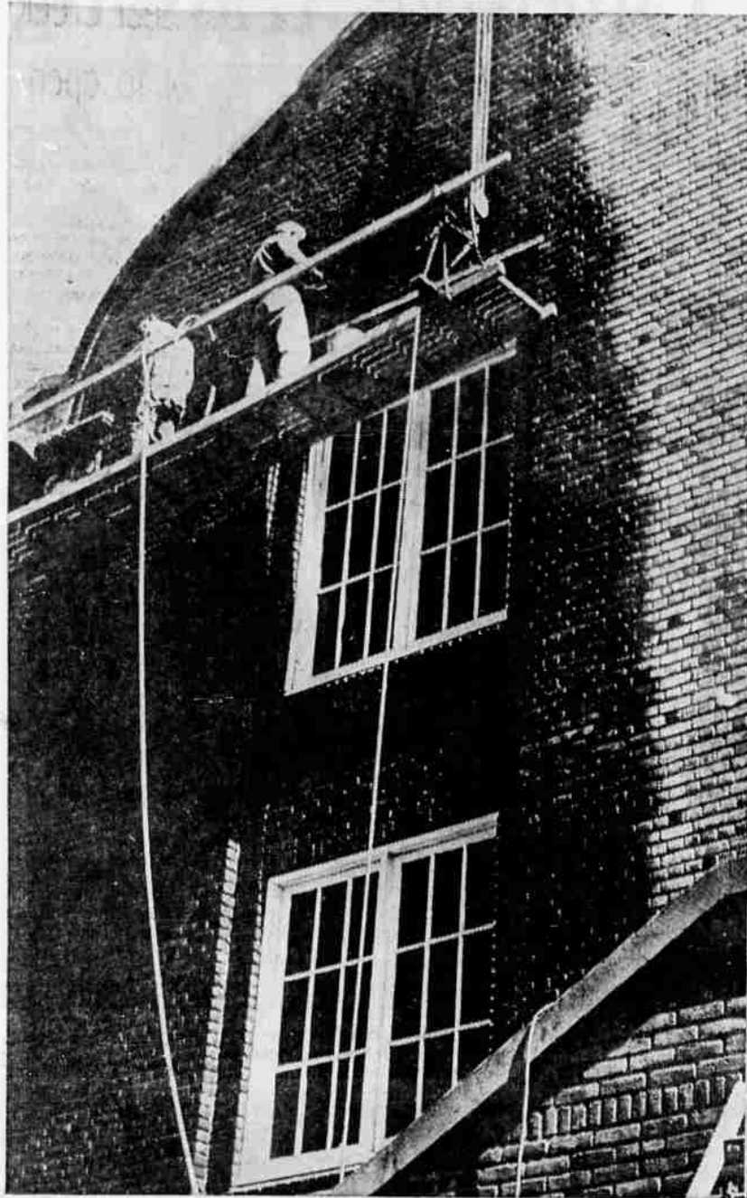
FACE LIFTING — Bend Junior High School is having its face lifted in preparation for the 1963-64 school year. Maintenance men have been replacing mortar in the brickwork by a process known as pointing. The crew has also put a new roof on Ried-Thompson School this summer.
