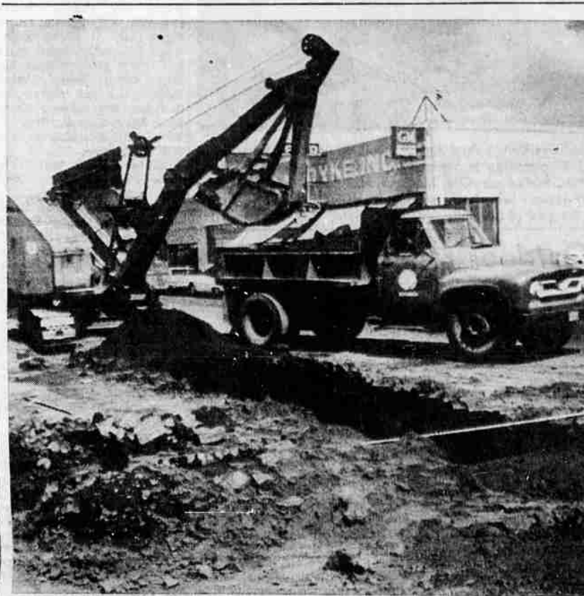
YARD-WIDE HOLE — City crews are pictured working on a yard-wide trench along Bond Street for a new 12-inch water main. The original pipe was installed in 1921. Crews are expected to complete the Greenwood to Franklin project in about one month.
