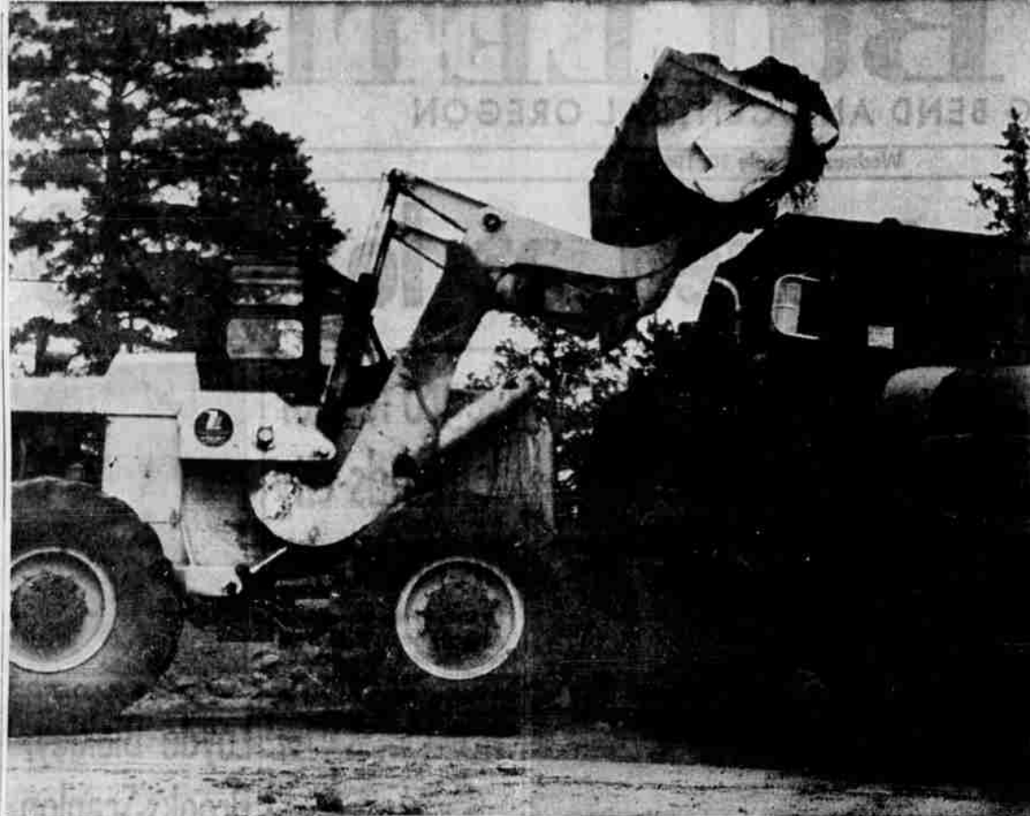
PAVING UNDERWAY —Dump truck takes load of dirt from county power shovel in first phase of dirt-street paving operation at West 11th and Quimby. At least three other dirt roadways in Bend are scheduled to undergo paving in 1963.
