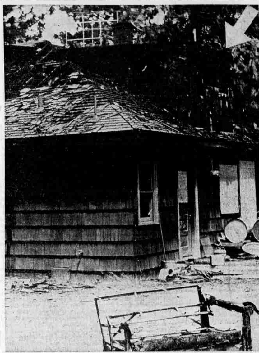
DEATH FIRE — Arrow points to north bedroom of Sisters sporting goods store loft where proprietor Lewis E. Johnson died when fire gutted building early Sunday morning. Three fire rigs and fourteen firemen battled blaze for an hour and a half. Mr. Johnson had been sole owner and operator of establishment for several years.
