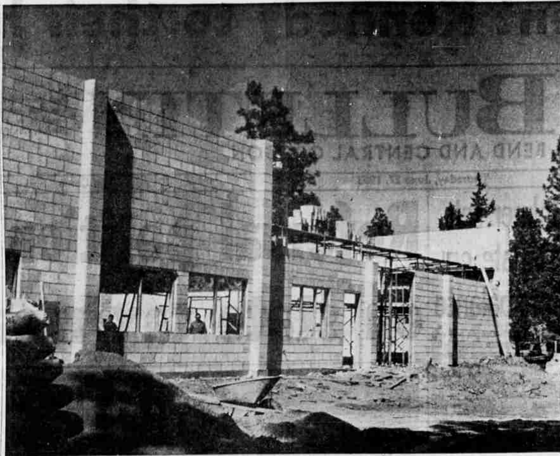
GOING UP—The vocational arts section of the new addition to the Bend Senior High School is rapidly taking shape on the south side of the school. Plans call for the new area to be open for classes in late fall. DeGree Construction Company of Bend is the general contractor for both the high school addition and the new Bear Creek Elementary School.
