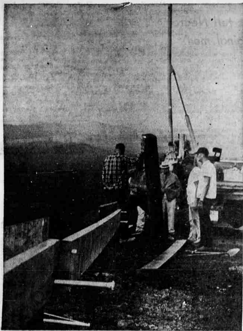
LAVA BUTTE GETS GUARD RAILS —Under construction at Lava Butte, adjacent to U.S. Highway 97 some ten miles south of Bend, is a guard rail, on the outer side of the spiral road leading to the butte top. This is a view west, with the contracting crew at work on the mile-long project.
