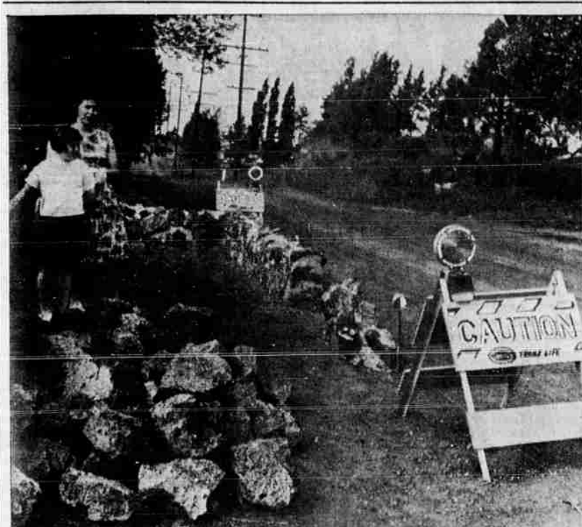
CITY HEADACHE—Proving great problem for City of Bend is this rock wall being constructed by Robert D. Reif, 1559 Division. Reif's wall is designed to protect his property, but police fear its potential danger to motorists. City may buy some of Reif's front property, but hasn't had an offer from him yet. Pictured are Mrs. Reif and ten-year-old daughter Marilyn.
