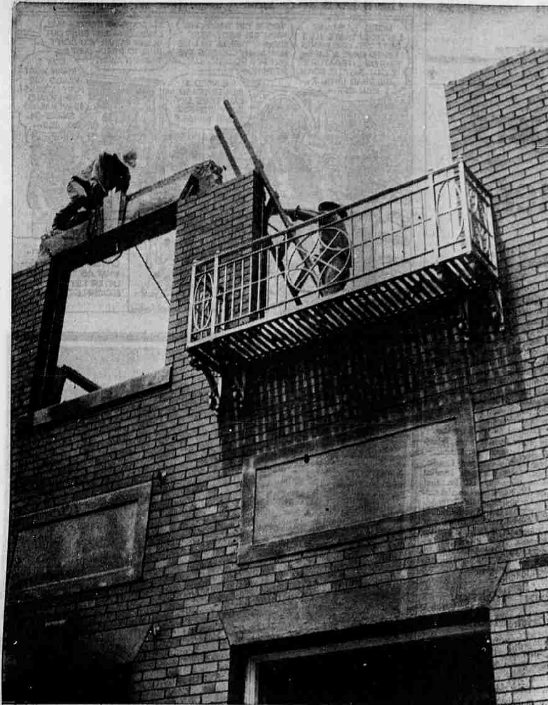
LANDMARK FALLING FAST—The old U.S. National Bank building in Bend is being razed for parking area. The bank recently moved into a new building. The old bank was built in 1912 and was a branch of U.S. National since 1946. The original name was the First National Bank of Bend and was run by C. S. Hudson.
