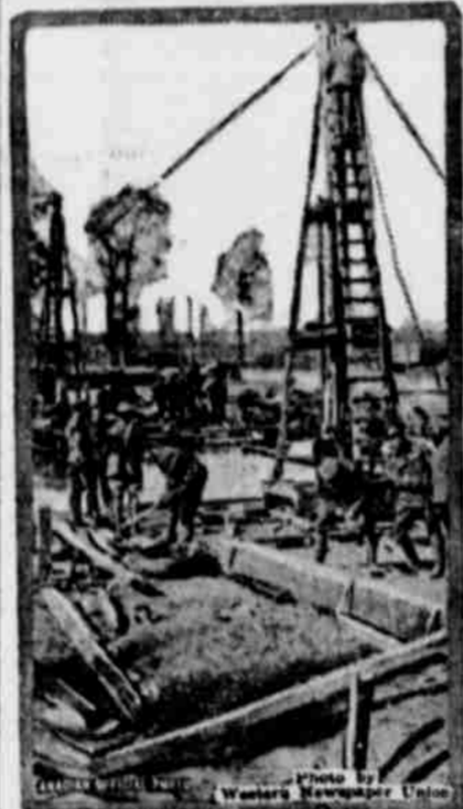
This Canadian official photograph shows the kind of work that must be done in France. These Canadian engineers are building an extra bridge across the Canal du Nord. A bridge in the right was built by these engineers in eight hours under heavy shell fire.
