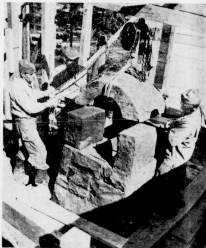
This unusual photograph shows the final stone being lowered into place on one of the huge chimneys which serve the new Officer's Club. These trainees, who are engaged in heavy construction, work under the guidance of the Specialist Branch.
