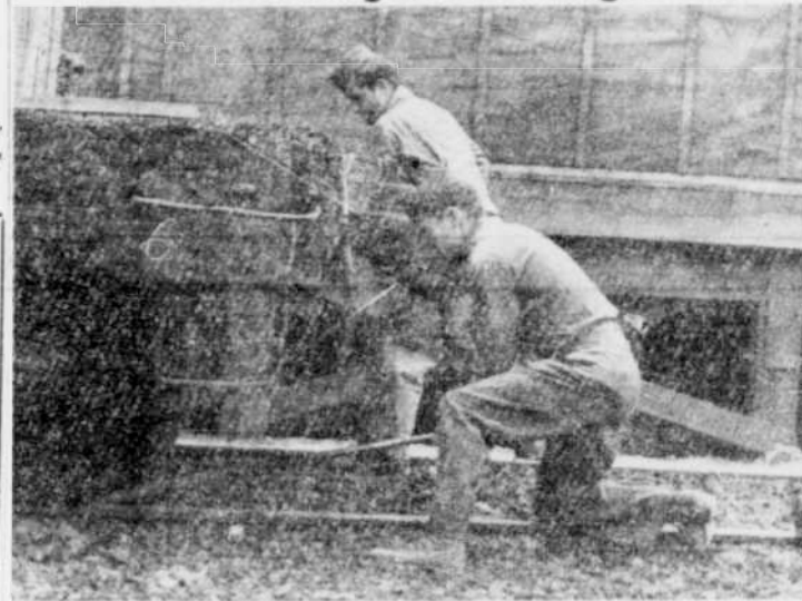
NOT A FAKE SHOT —When the ERTC was emerging from its construction stage, facilities for unloading and moving railroad cars were unobtainable. As a result, these two Abbotmen, first ERTC'ers to land here, had to do plenty of rugged work by brain and brawn. M/Sgt. Bill V. Anthony and Sgt. Tommy Simerlink show how they used to move r. r. cars. Looks easy, well, it isn't! (ENGINEER Photo by Hahn).
