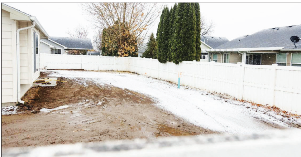
This backyard in Fruitland, pictured on Thursday, Dec. 1, 2022, was excavated to search for human remains related to the missing child case of Michael Vaughan.
