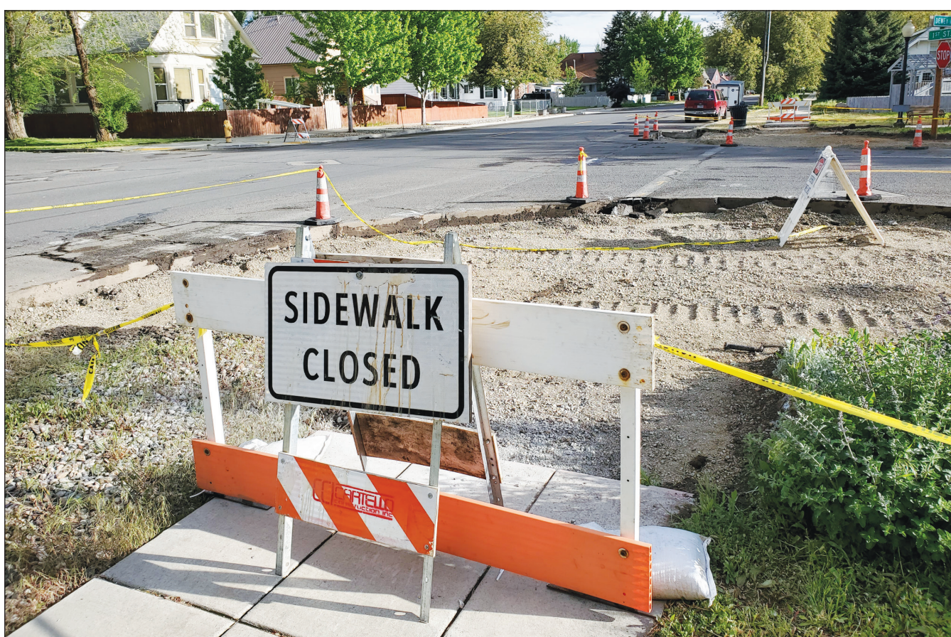
Work was underway on June 2, 2022, on a wheelchair-accessible curb ramp on Dewey Avenue near Estes Street in Baker City.
