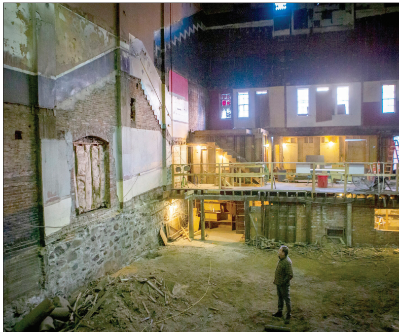
Ben Lonergan/East Oregonian Rivoli Restoration Coalition President Andrew Picken looks at the brickwork Tuesday, Dec. 14, 2021, where a former beam spanned the interior of the Rivoli Theater in Pendleton. Developer Parley Pearce is using parts of the 50-foot beam in the Oak Hotel, the former brothel in downtown Pendleton he plans to open as a boutique hotel.
