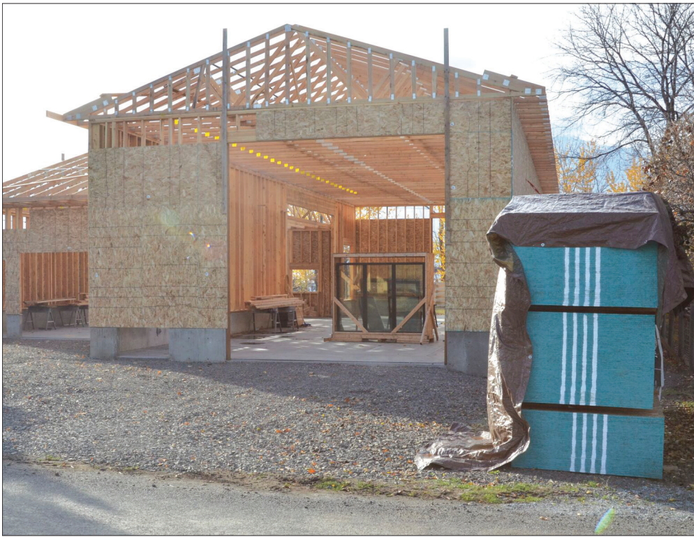
Bill Bradshaw/Wallowa County Chieftain New windows and a stack of expensive plywood wait to be installed at a new house under construction on Mill Street in Joseph on Tuesday, Nov. 2, 2021.
