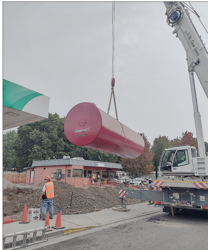
Contractors prepare to install a new gas tank at the Falk's Mini Mart gas station in Union on Wednesday, Sept. 8, 2021.
