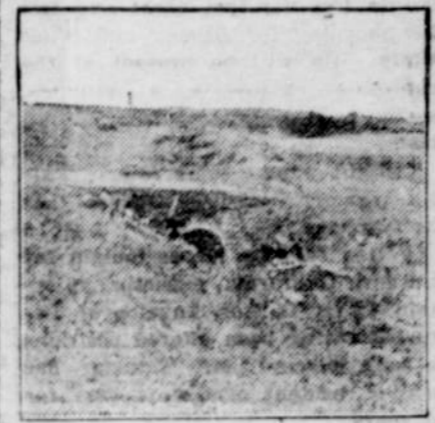
Method of Carrying Terrace Water Under a Roadway by Means of a Culvert.
