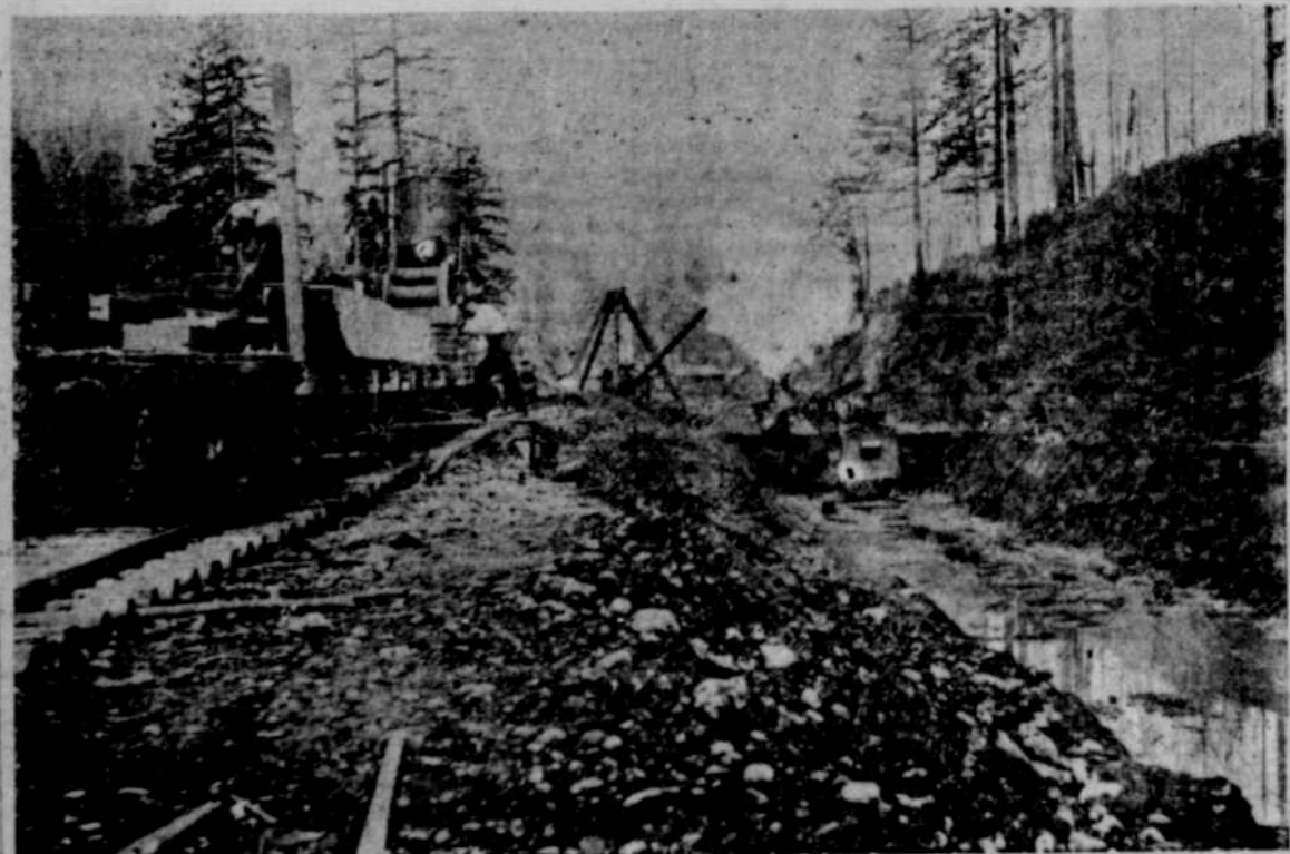
STEAM SHOVEL EXCAVATING CANAL CONNECTING DAM WITH LARGE RESERVOIR AT O. W. P. ELECTRIC POWER PLANT.
