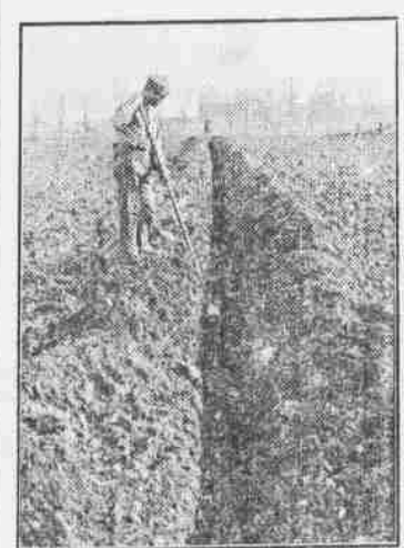
POOR WAY TO LAY TILE
