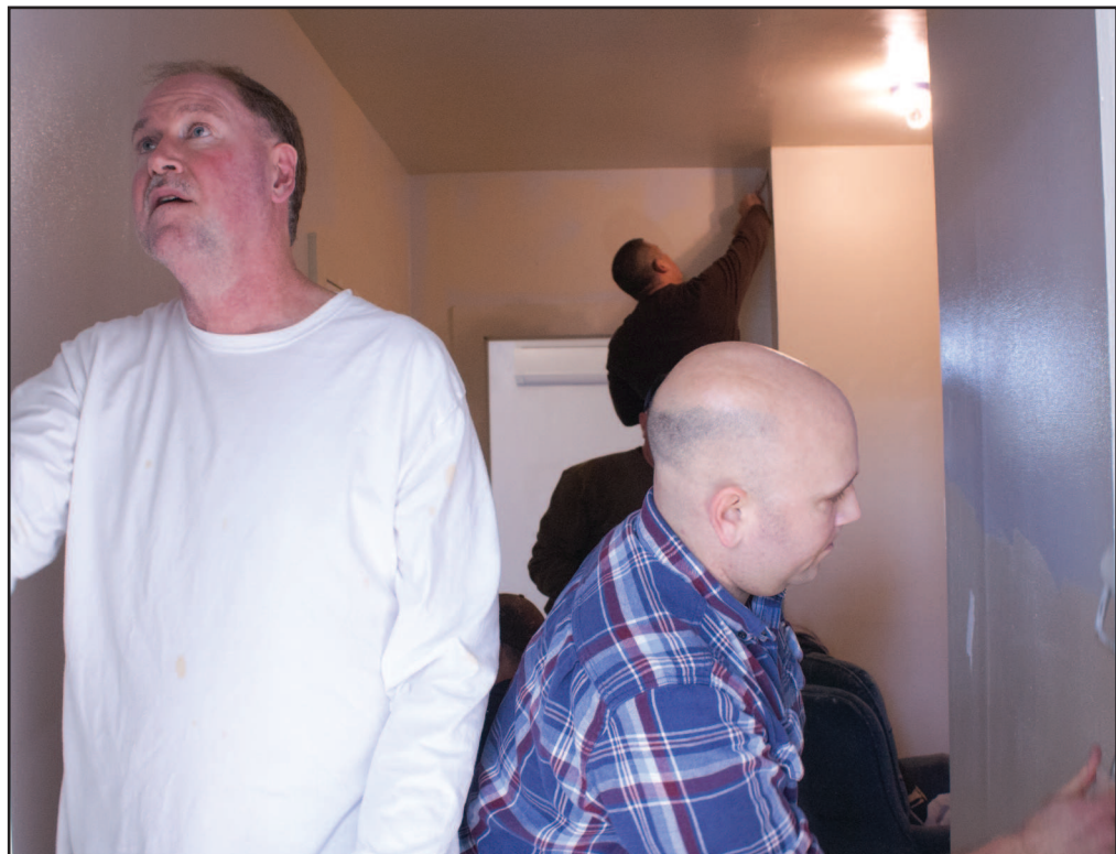
Deputies John Kincaid, left, and Matt Garrett paint the hallway at Titus 3 House in Dallas on Saturday. The Polk County Sheriff's Office volunteered to help with the project.
