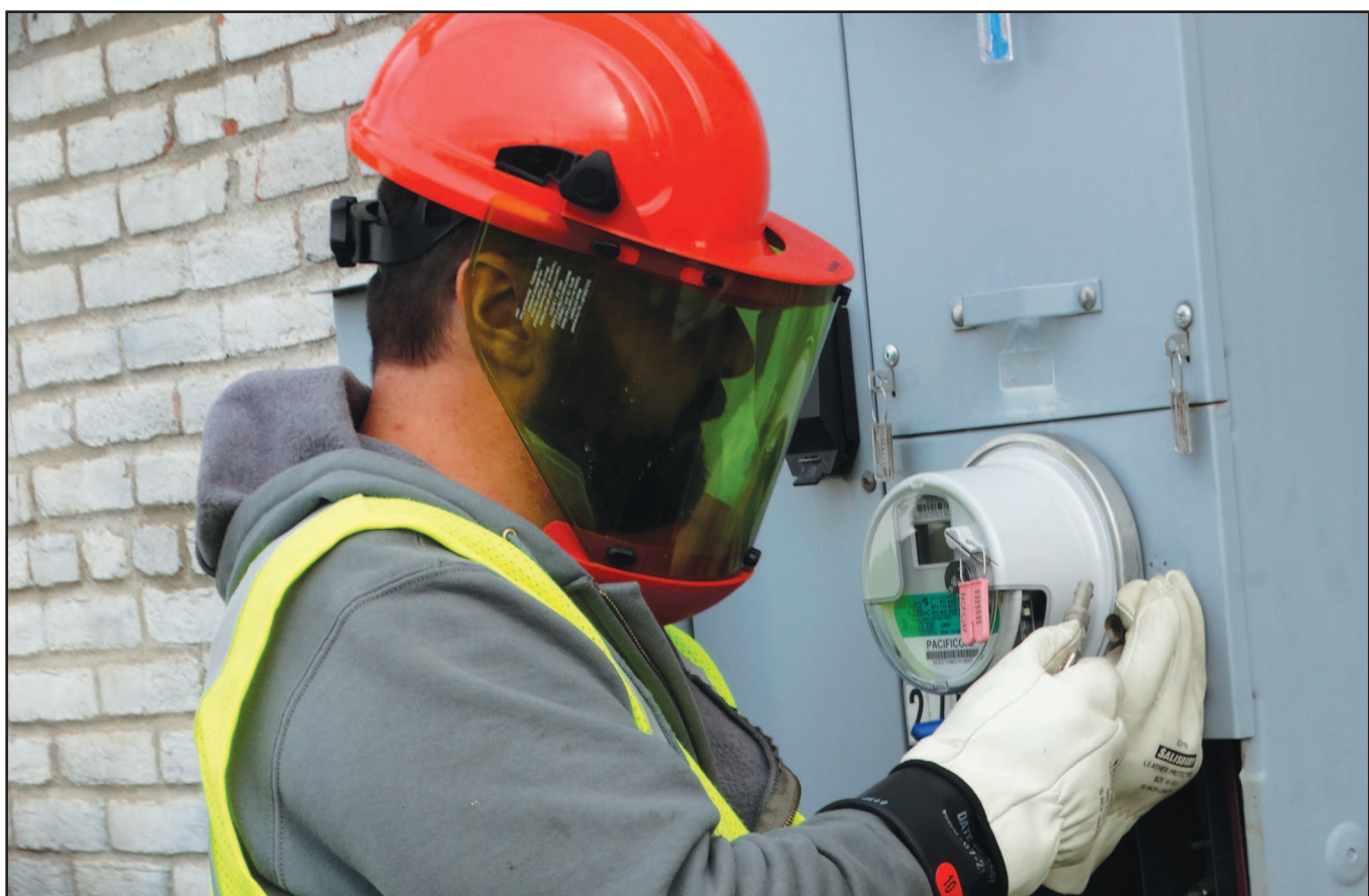
John Sanders, Pacific Power field supervisor, installs a new smart meter at Indy Commons in Independence.
