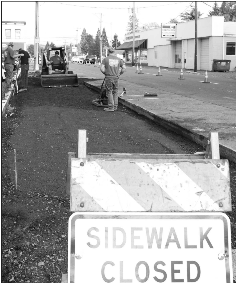
A Liberty Concrete crew prepares the sidewalk for paving on Jefferson Street by the Polk County Courthouse. The project is part of a Dallas Urban Renewal "streetscape." Polk County will repave the Court and Mill streets sidewalks on the courthouse square.
