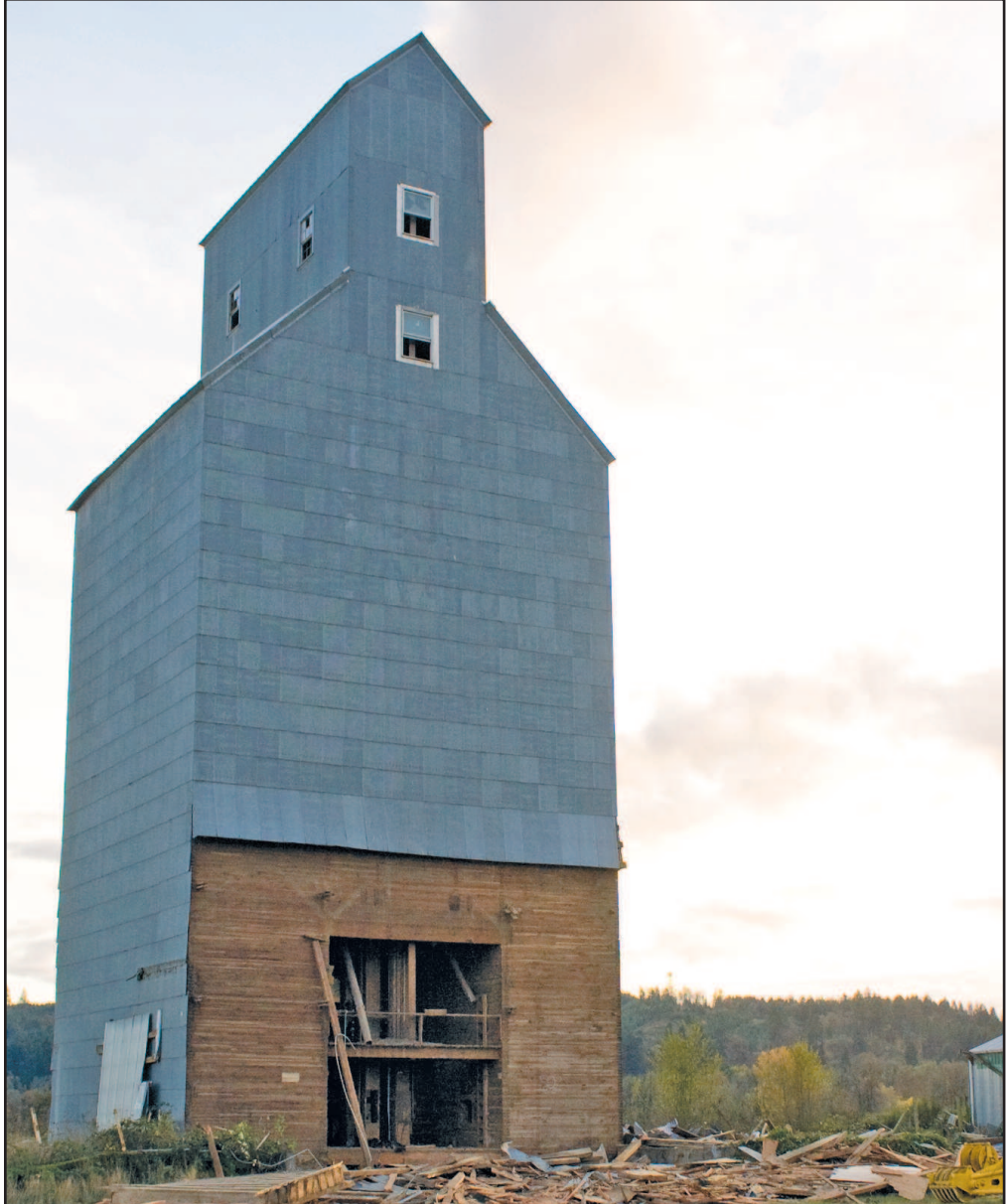
Crew began tearing down the grain elevator on property owned by Valley Life Center last week. The building has fallen into disrepair and considered a safety hazard.
