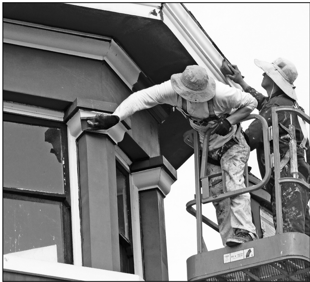
Workers sand the tower on Friday morning at the Cooper Building in Independence and cover some sections with primer. The building is getting ready to be painted a traditional blue-gray. The building has been under construction during restoration.
