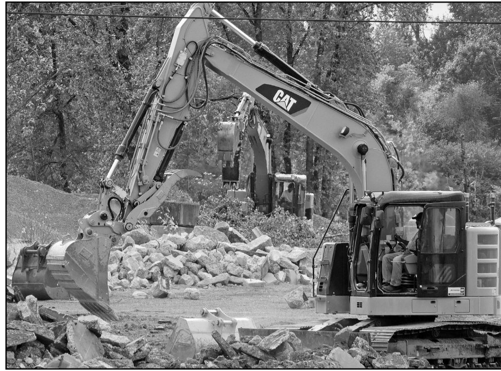
Demolition continues as workers make the old Valley Concrete site on the Willamette River shovel-ready for whichever developer the city decides to sell it to.
