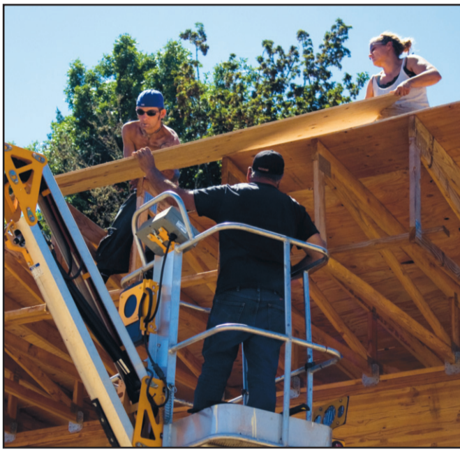
JOLENE GUZMAN/Itemizer-Observer Workers with Robert Young Construction place a board on the roof of the new cover over the stadium at Falls City High School's football field on Friday.
