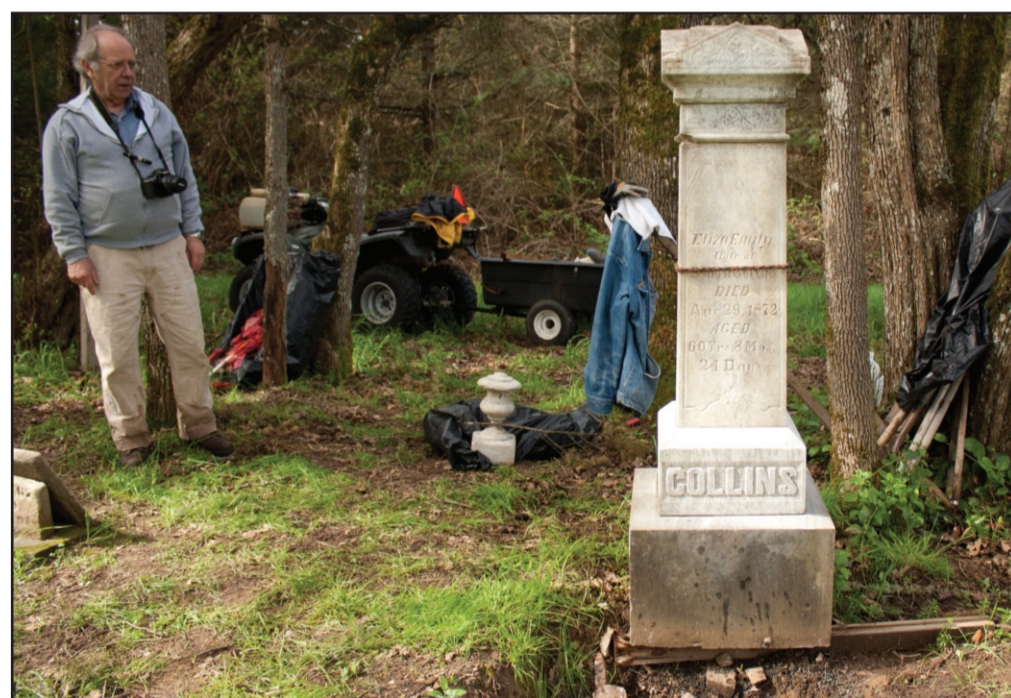
JOLENE GUZMAN/Itemizer-ObsERVER Collins examines a monument that will have to be repaired and repositioned in its original place. Finishing the job will require pouring a new base and sliding it into place.
