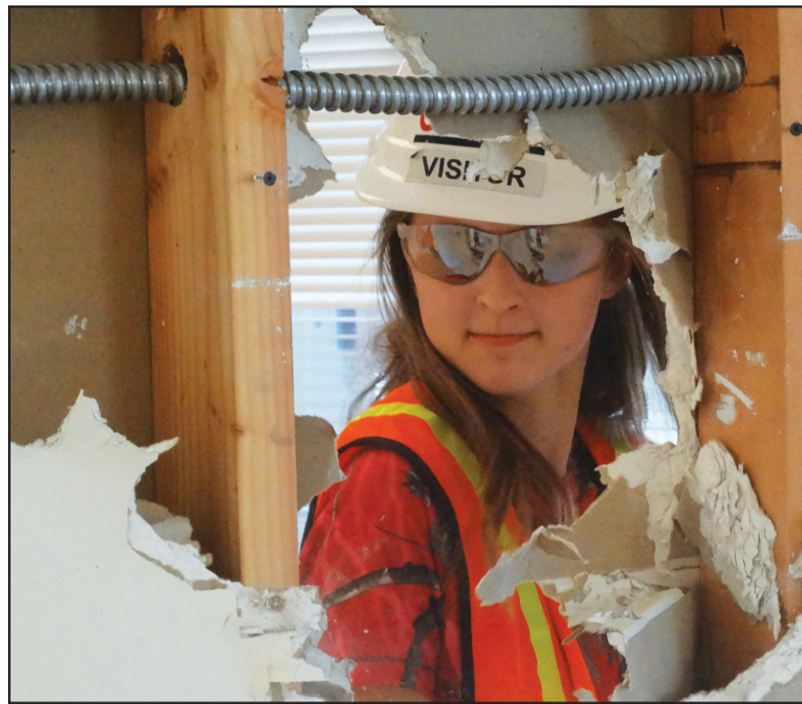
Central Student Sarah Hall helps tear down walls after school on Thursday in what will be the child development area at the health center.
