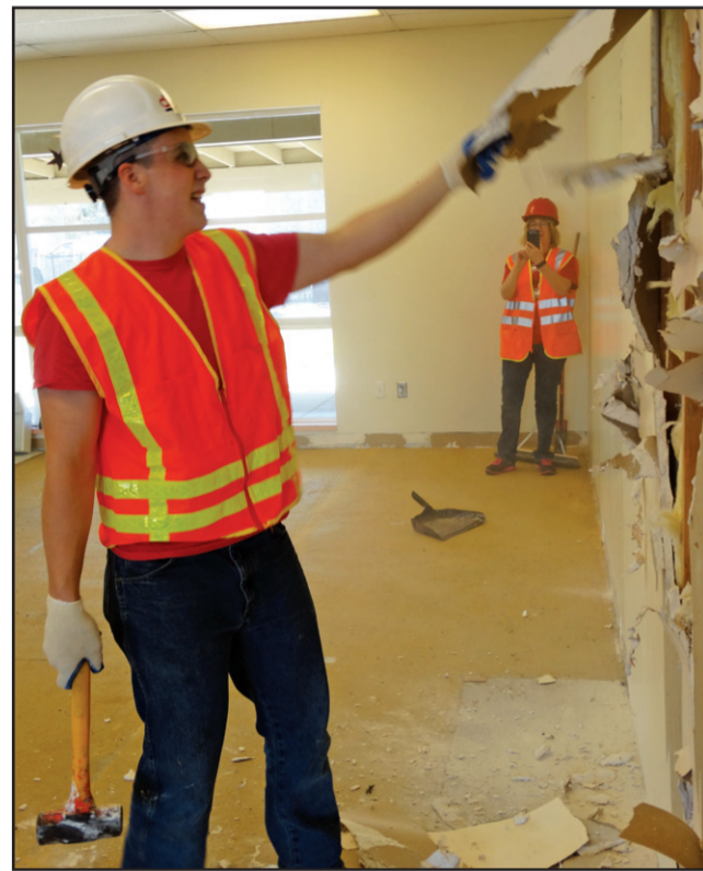
EMILY MENTZER/Itemizer-Observer Central Student Jaron Timshel rips out sheet rock and insulation at what will be the Central Health and Wellness Center on Thursday. The center will open in June.
