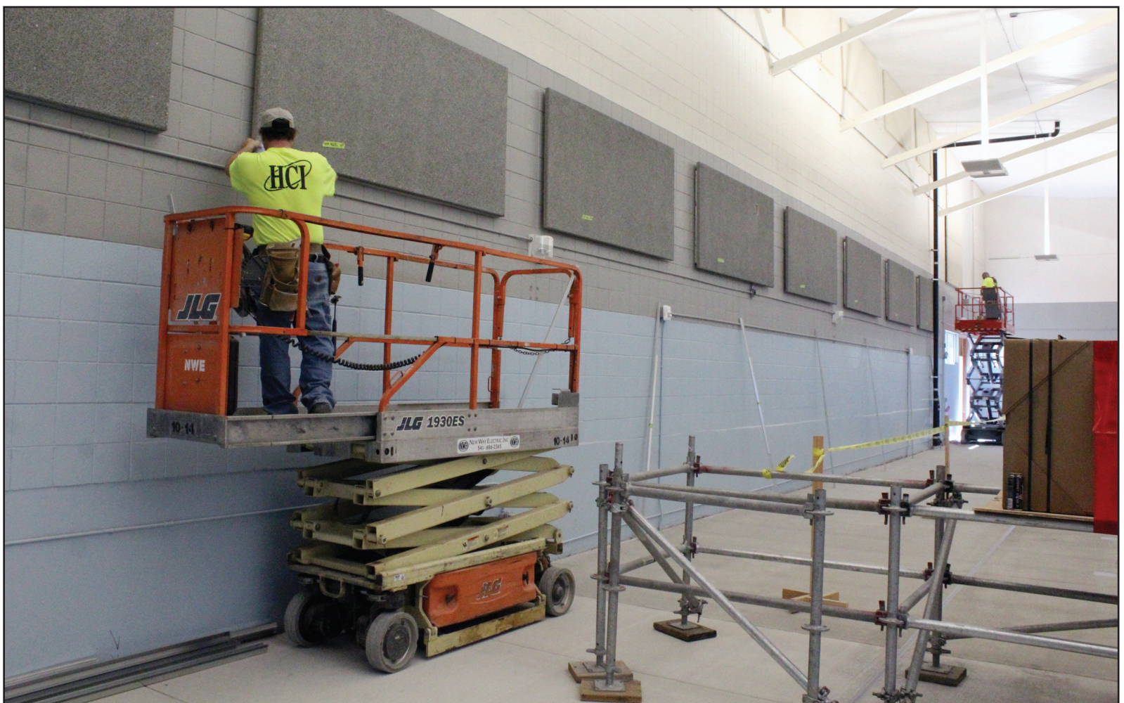
A worker installs tectum panels, to ensure there is little to no echo in the space, at the Warren H. Daugherty Aquatics Center last week. The center is undergoing a renovation process that will be completed in the coming weeks. PHOTO BY ZACH SILVA/CG SENTINEL
