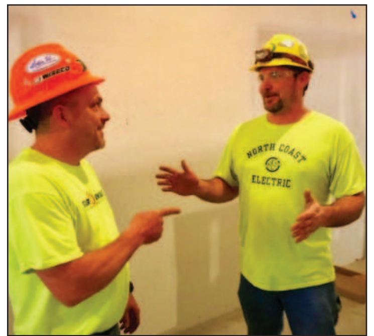
South Lane School District Project Manager Matt Allen (left) jokes around at the end of the work day with Michael Cordin, a Cottage Grove resident and electrician for the new Harrison Elementary School.
