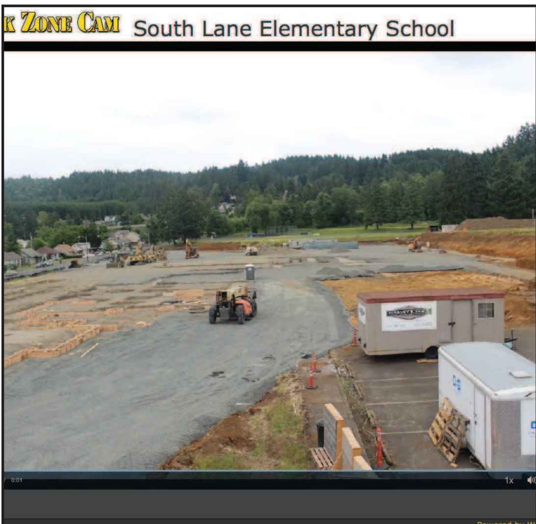
South Lane School District has installed timelapse cameras at the site of the new Harrison Elementary School on Taylor Ave. To check in on the progress, follow the link and see the activities surrounding the construction. http://www.workzonecam.com/projects/southlane/southlane/workzonecam
