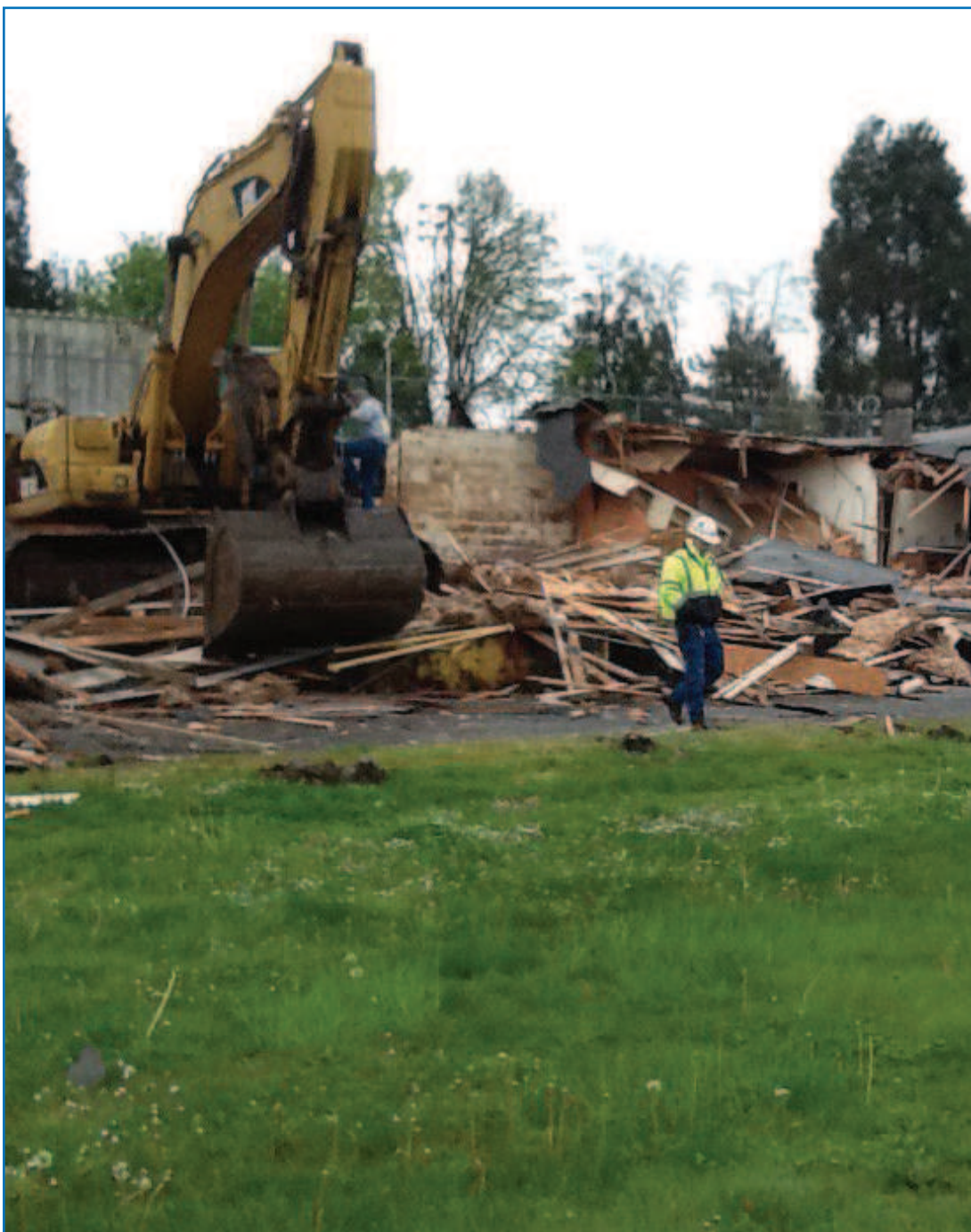
The new Harrison Elementary School on Taylor Ave. is scheduled to be ready to receive students by Fall 2018. Demolition on the project started late last month with accessory buildings being torn down and initial plans underway. The school is set to house nearly double the number of students the current elementary school houses and has been designed with Pacific Northwest features, a new library and cafeteria space. Colors will guide students to the proper grade-level areas and final estimates have the school's construction costs clocking in at roughly $22 million. Photo courtesy South Lane School District.
