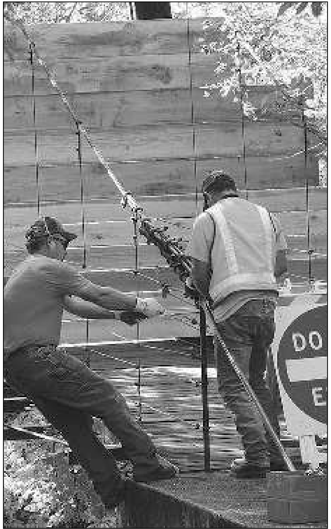
City workers secure the Swinging Bridge at the end of last year after it was deemed to be dangerous to remain open to the public. Residents will now be able to contribute to its repair by rounding up their water bills with the funds going into a trust fund for the bridge's repair.
