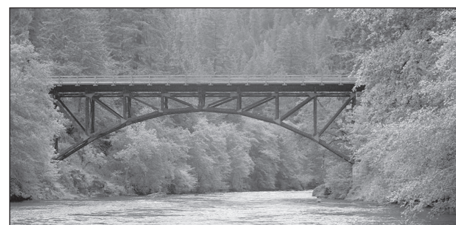
Inspection of the Mott Bridge on the North Umpqua River is expected to cause significant delays July 7.
