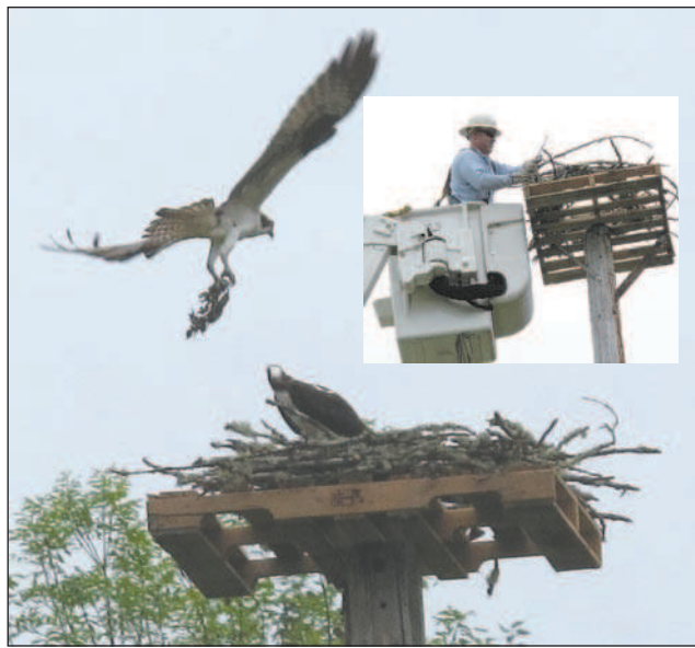
In the inset, EPUD serviceman Neil Williamson installs a new osprey nesting platform, which the birds soon occupied.
