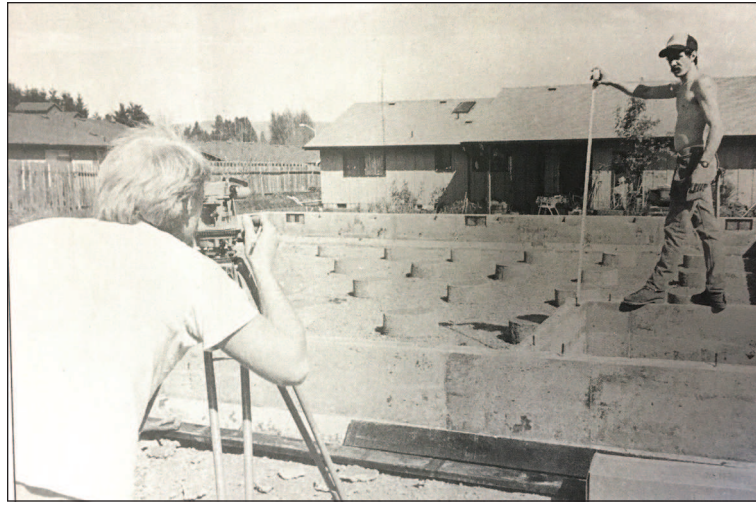
Construction workers Bruce Bergby and Terry Hughes check foundation level at housing start on Jason Lee Avenue.
