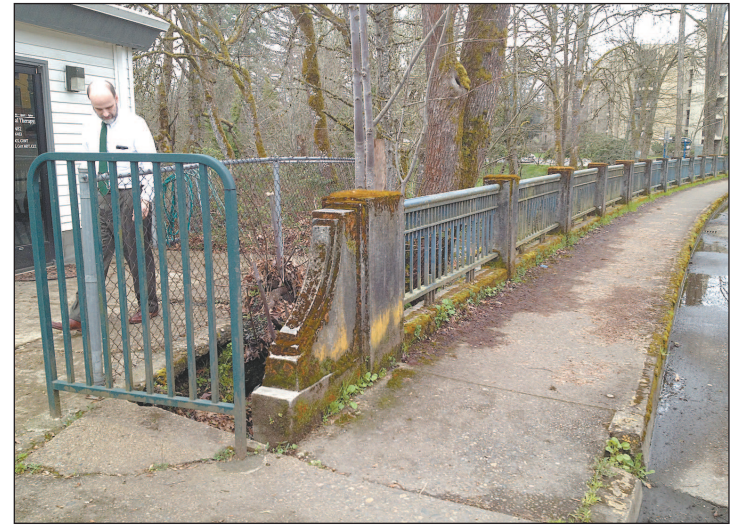
City Manager Richard Meyers examines evidence that the ground under a downtown bridge is washing away.
