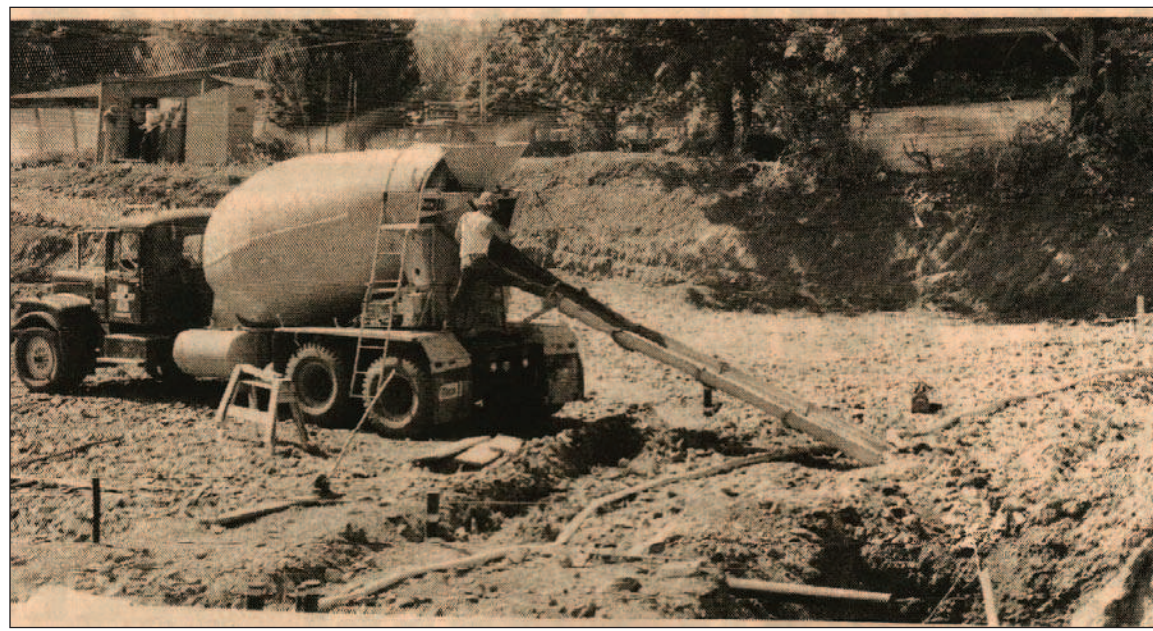
Sept. 18, 1975: CG launches City Hall project — Area residents who have waited for some time for signs of construction activity at the Main Street site of Cottage Grove's proposed City Hall got a treat last week. Work crews at the site poured concrete for the first time and the concrete truck that delivered the first load nearly didn't make it out of the construction site.
