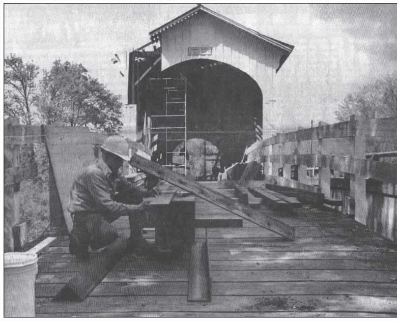
May 24, 1995: Minding the gap — Dick Krantz of T.G. Nelson Electric works on the Curin Bridge. The historical bridge is just one of several in the area that are undergoing major repairs.
