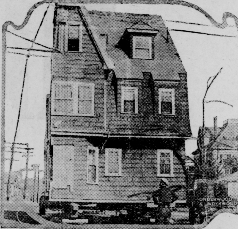
This half of a three-story house was photographed while being moved along Commonwealth avenue, Newton, Mass. The section, weighing approximately 40 tons, was being moved from the residential section of Newton to a site one-quarter of a mile from its original spot.
