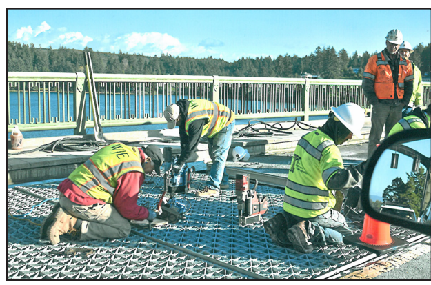
ODOT crews work on the new metal lift span decking on the Siuslaw River Bridge.
