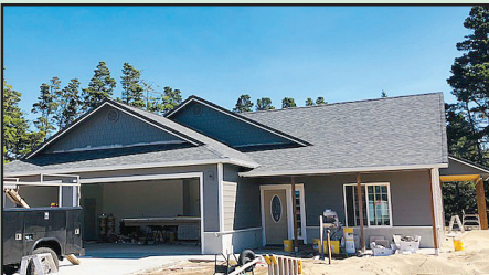
5225 Dunewood Dr – Beautiful, custom home currently under construction in the Reserve at Heceta Lake. Built by Ron Mann Construction. This 3 bdrm, 2 bath home with 2002 sqft boasts a 3-car garage, granite counters and a seasonal lake view. $679,000. #3263-21535037
