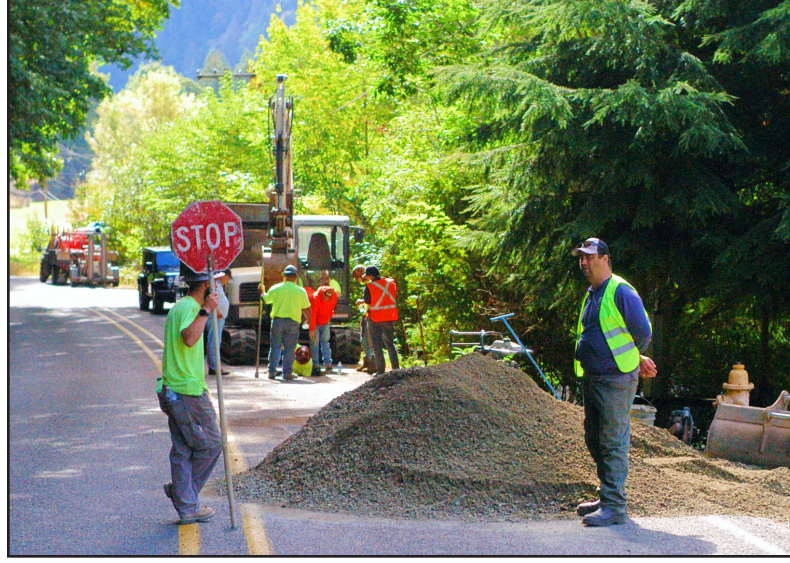
Workers from Delta Operations, of Eugene, assist Mapleton Water District workers on leak repairs on East Mapleton Road.
