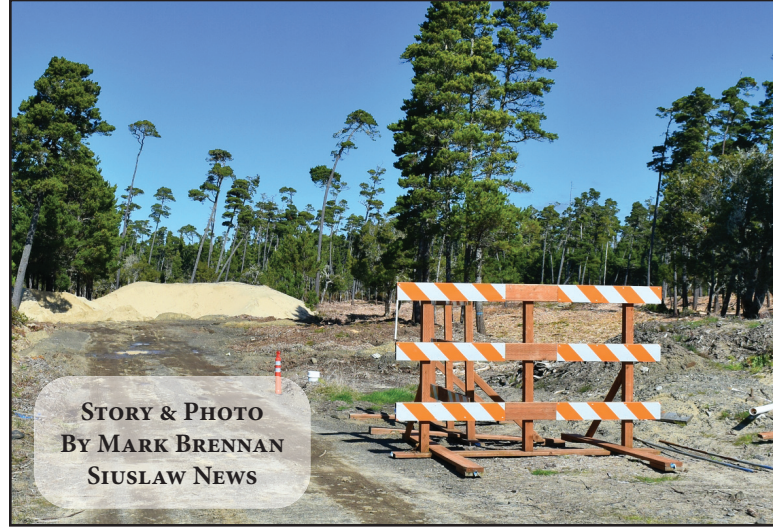
Pacific Golf Communities, LLC, has been fined by the City of Florence for construction work being done at Fairway Estates on Rhododendron Drive.
