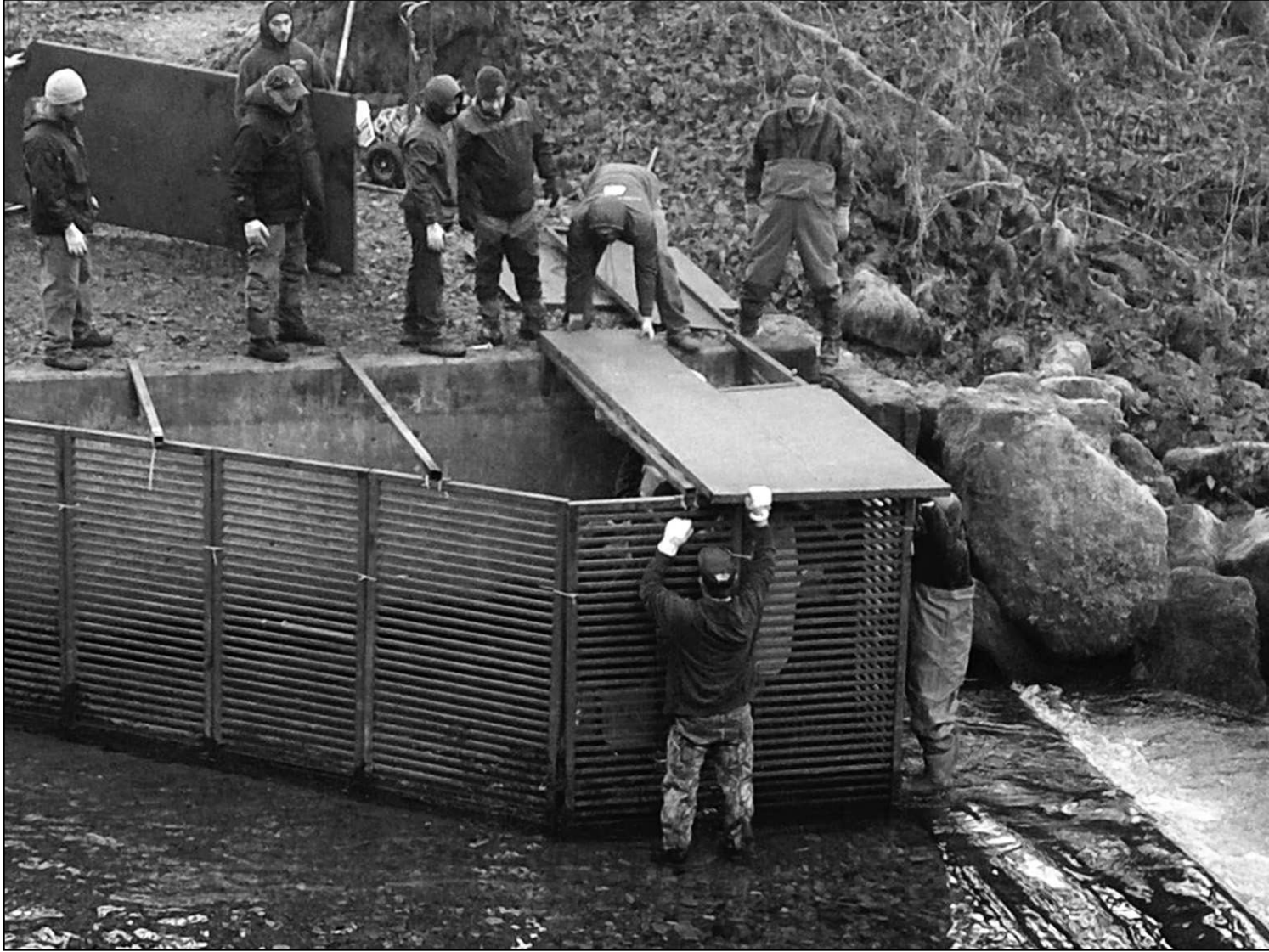
STEP volunteers and Camp Florence crew members help complete the installation of a salmon trap along Whittaker Creek in December.
