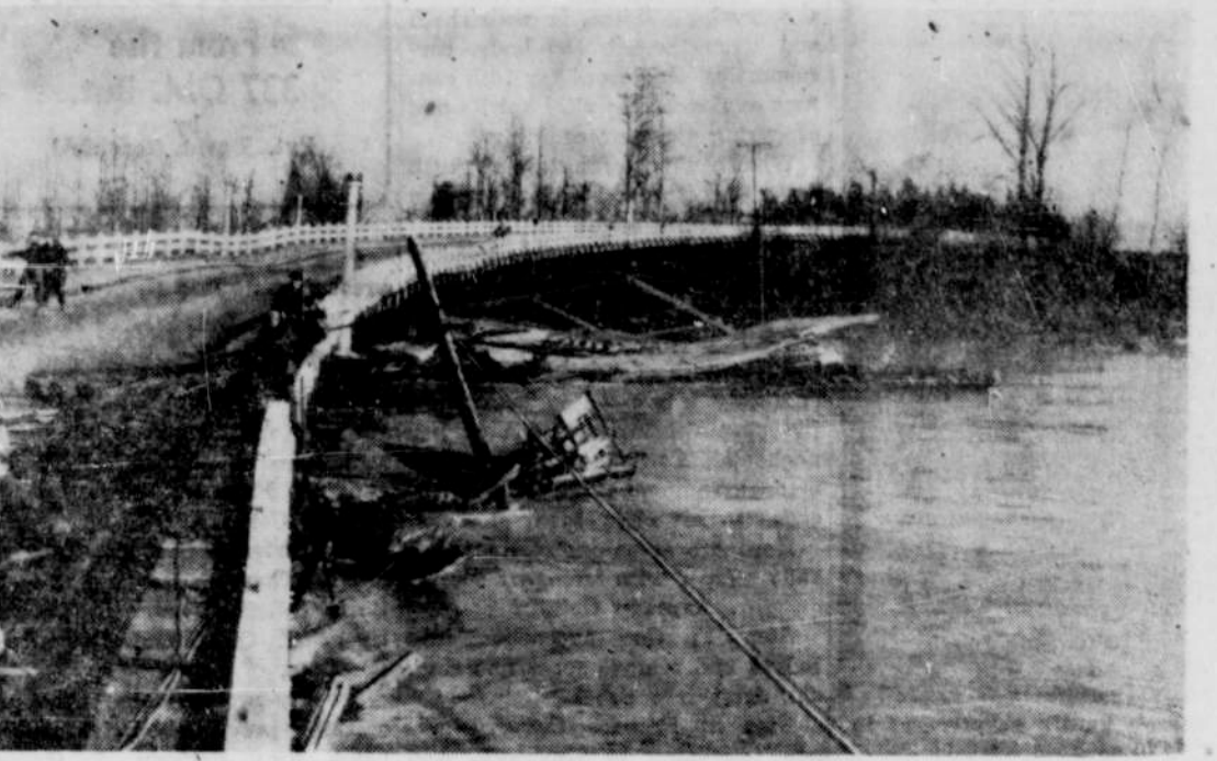
Once upon a time it rained and rained in Oregon. Proof is hereby presented in a photo that recently arrived by ox team. It shows the Mellow Moon dance hall and roller rink resting uncomformably under the West Salem bridge. The bridge has since been repaired. The Mellow Moon, alas, is no more.
