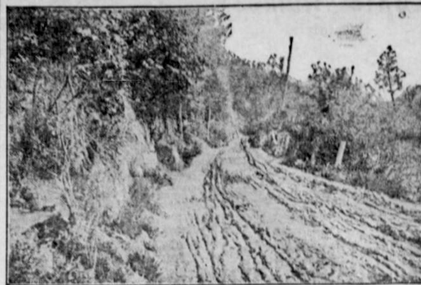
The illustration shows a strip of highway along the famous "Scogg River Narrows," in Tioga county, Pennsylvania, before it had been macadamized.
